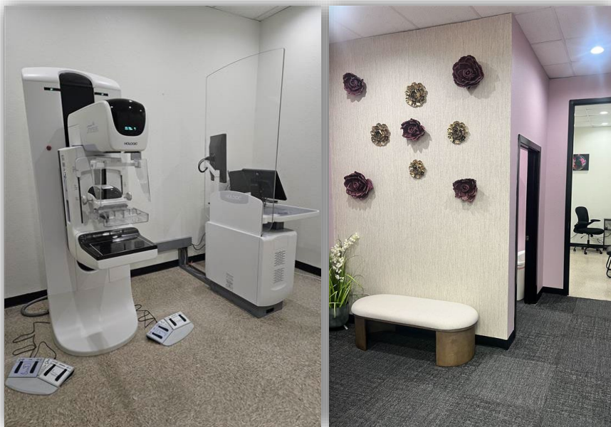
MyCHN's newly installed mammography unit and suite at the Pearland Family Health Center clinic site, supporting breast cancer screening services for patients in Brazoria County, Texas.
